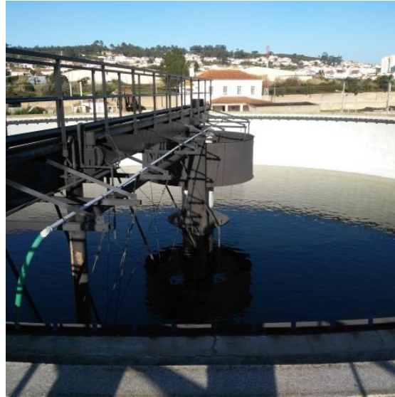
Figure vii. Secondary decantation tank.
