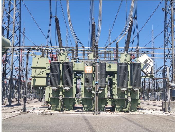
Figure 2.22: Power transformer at Paraimo substation.
