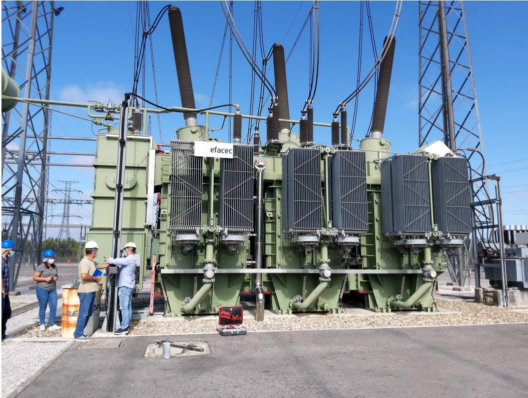
Figure 5.3: TRF6 power transformer. On the left, collaborators from REN working on the neutral cable of the transformer where the GIC measurement system was installed.
