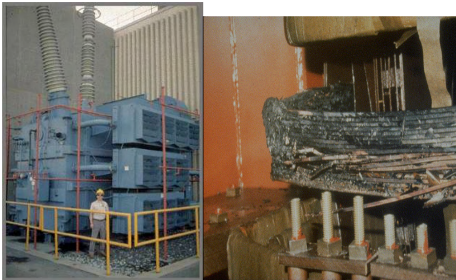
Figure 2.14: Damaged transformer owned by the Public Service Electric and Gas Company of New Jersey damaged by the March 13-14 th , 1989 geomagnetic storm. From Marusek (2007).
