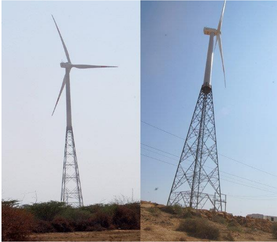
Figure 2.7 – Suzlon Energy 120 m hybrid lattice-steel tower
