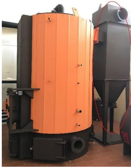
Figure 2.7. Multiple cyclone system (red circle) installed on the boiler system.
