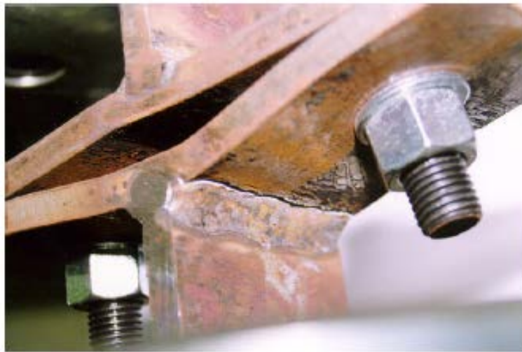
Figure 2.2: Failure mode of specimen under cyclic tests [8]
