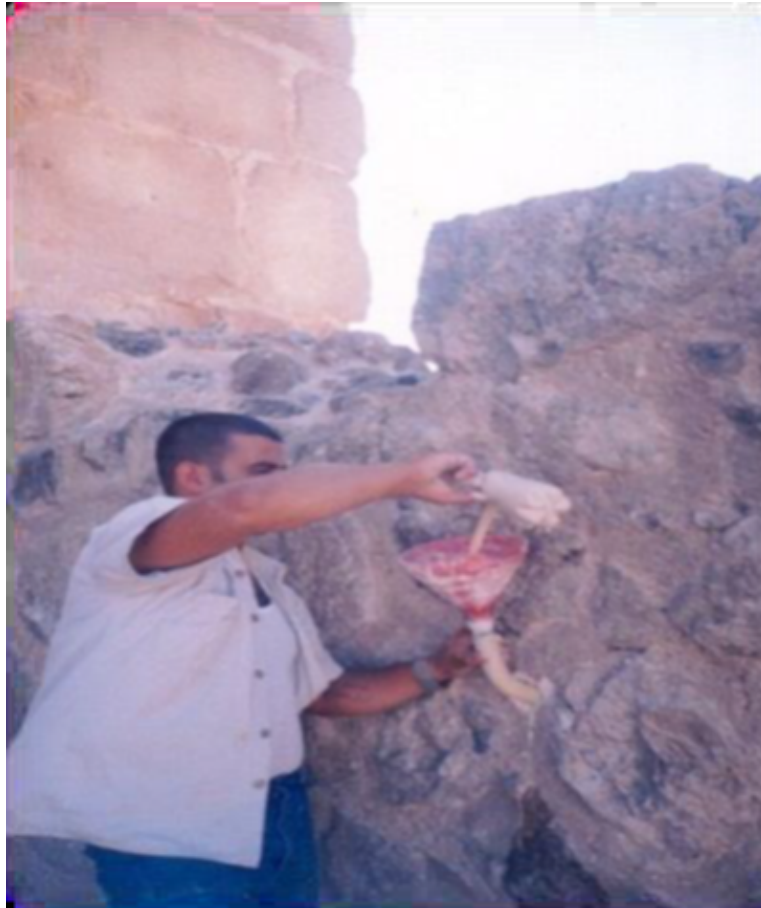
Figure: 12, injecting a new mortar into the spaces inside the wall (AKTC, 2007)
