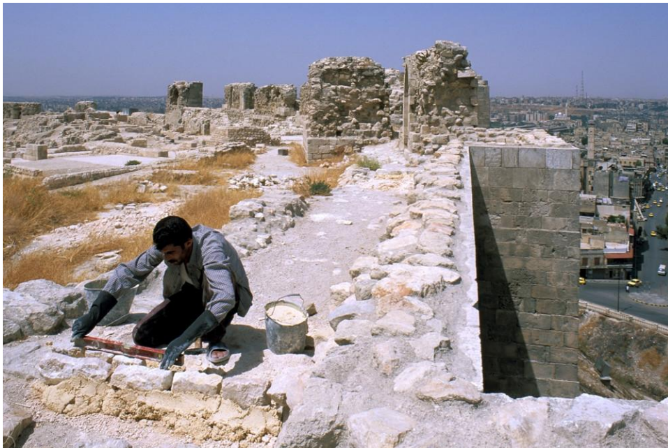
Figure: 13, injecting a new mortar into the spaces inside the wall (AKTC, 2007)
