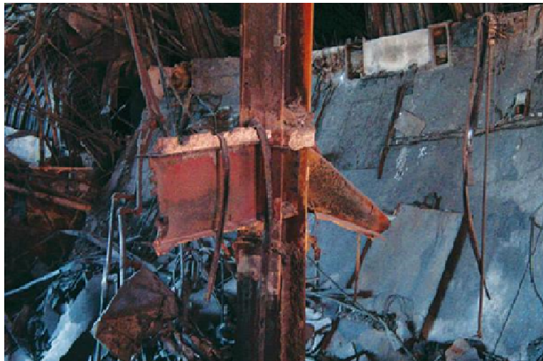
Figure 2.7. Connection failure in building 5 of The World Trade Center [65]
