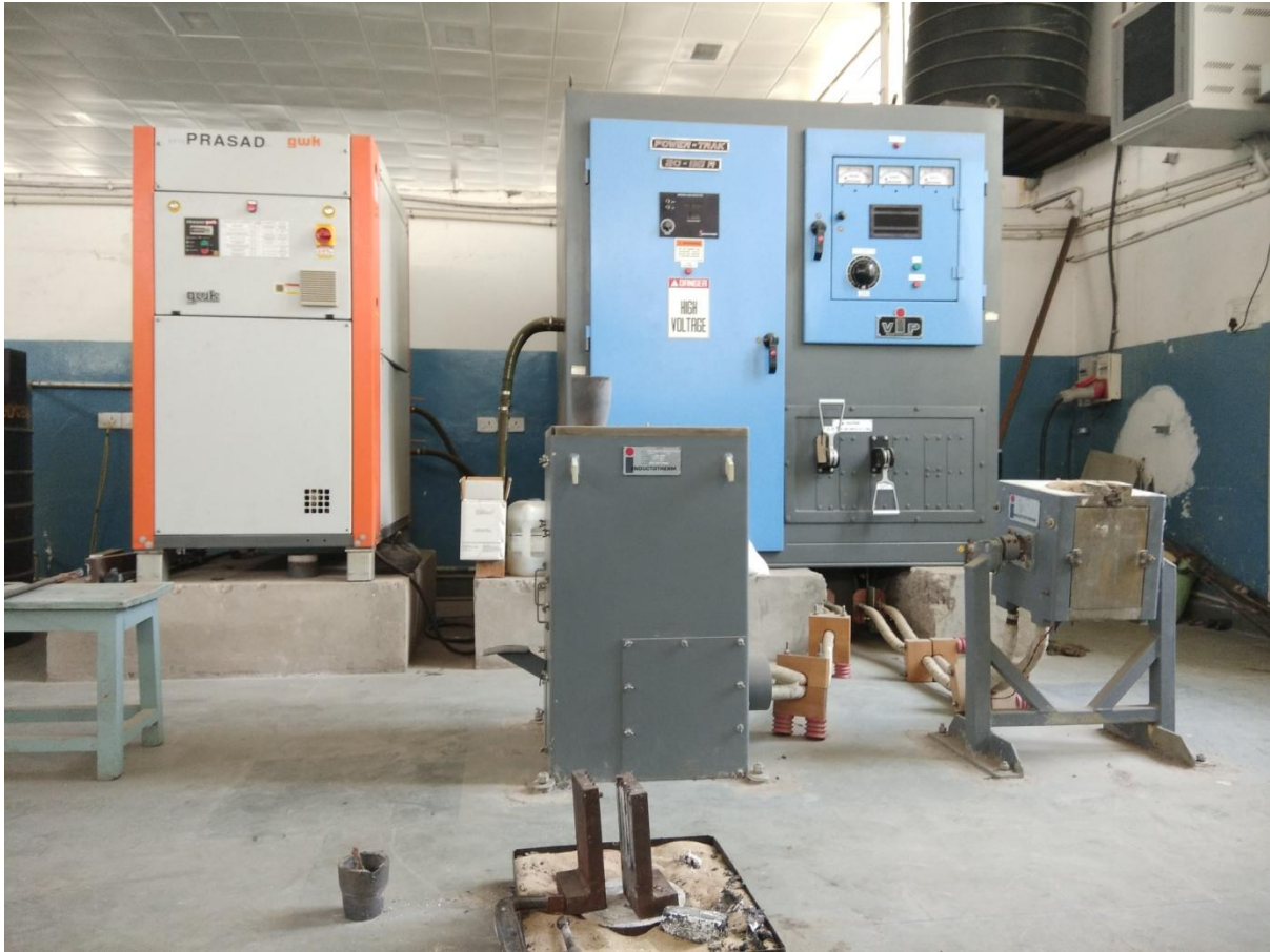
Fig. 11: Setup of Induction furnace with chillar
