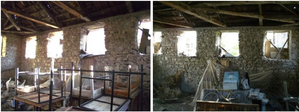
Figure 6 - Misuse of Green Island Bath
