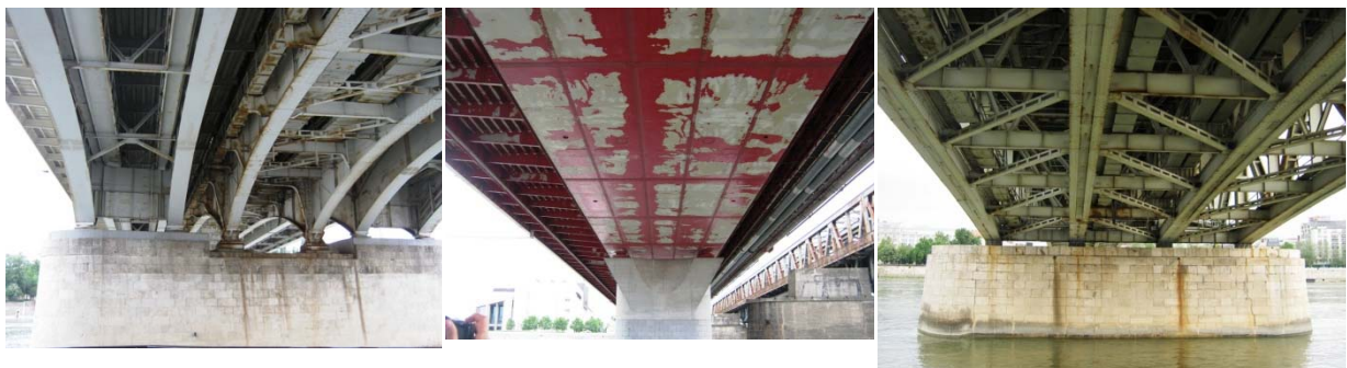
Figure 1.2 Corroded steel bridges in Budapest, Hungary; from the left to the right: Árpád bridge, Lágymányosi bridge and Petőfi bridge
