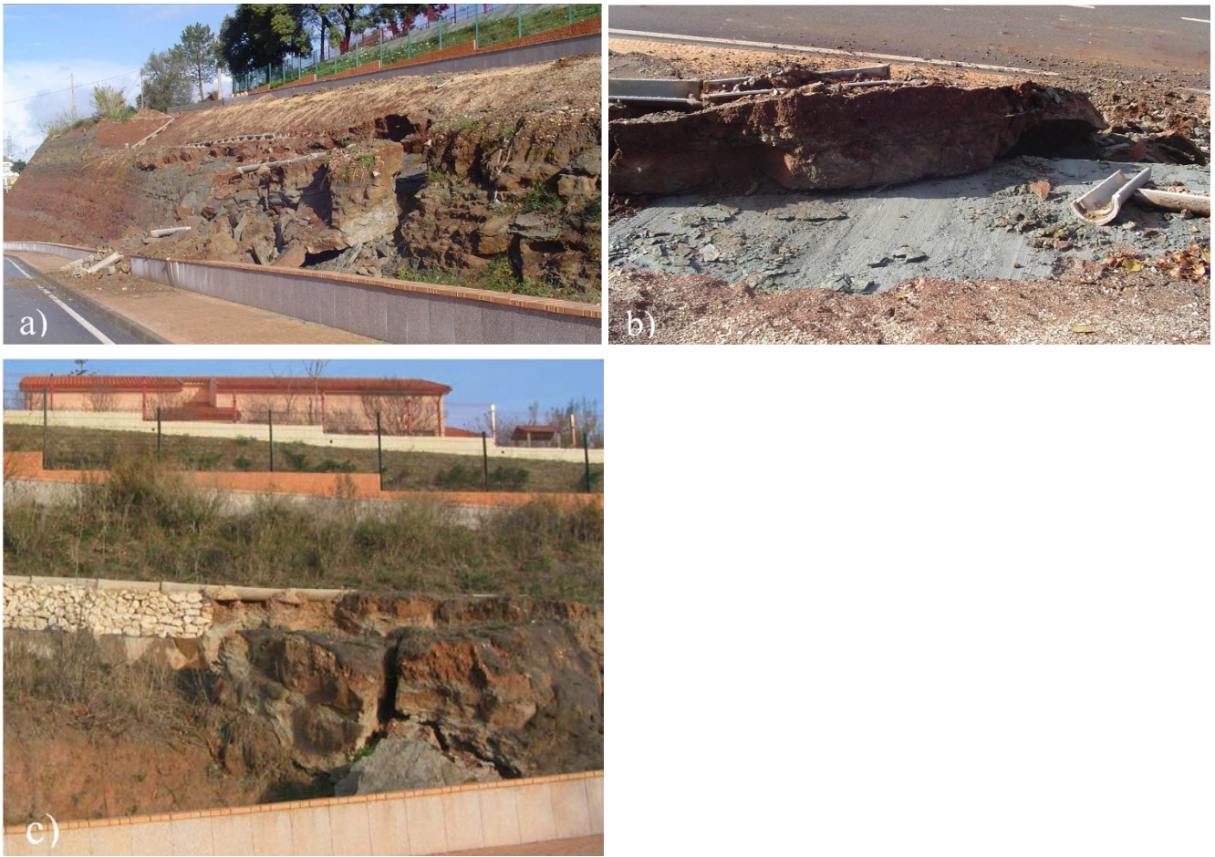
Fig. 4 Planar failures in the Areiro School slope. December 2005: a landslide occurred along the mudstone stratification, b slid block and slickenlines on the mudstone bedding plane. December 2007: c reactivation of the failure to the right of the 2005 slide
