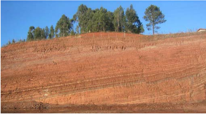
Fig. 8 View of the west cut slope of Quinta da Portela, around 20 m high, without any major instability features
