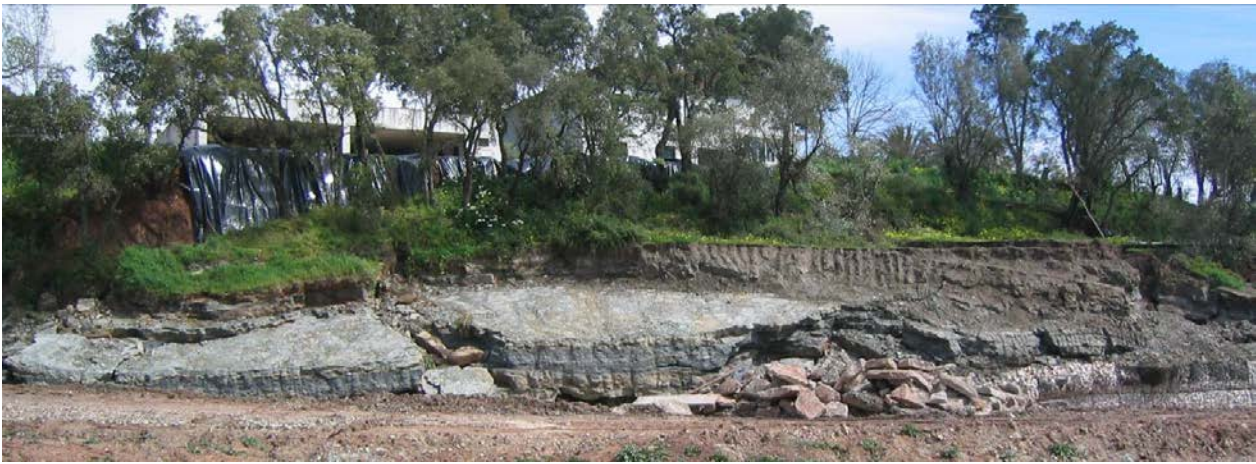
Fig. 5 Overview of the failed slope of “Quinta do Areiro” (March 2006). The black plastic liner in the background highlights the fault scarp oriented N48°W, subvertical, revealed by the slide
