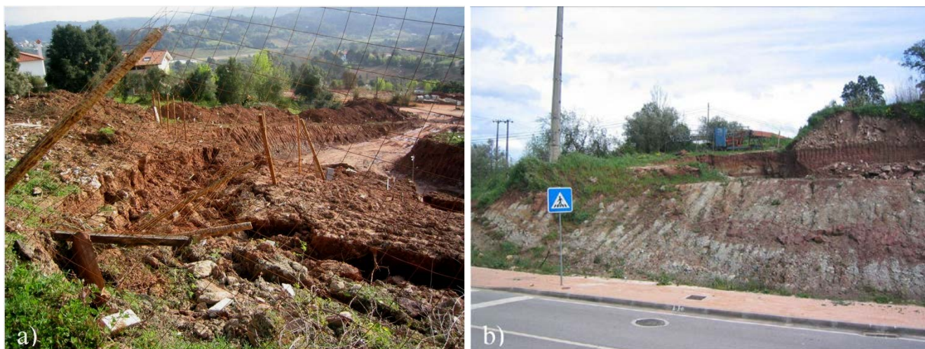
Fig. 3 Slide of the street to “Quinta do Areeiro” cut slope: a planar slide following excavation during construction, at the end of February 2004 and b geometry of the slope after removal of the failed ground, and final reshaping
