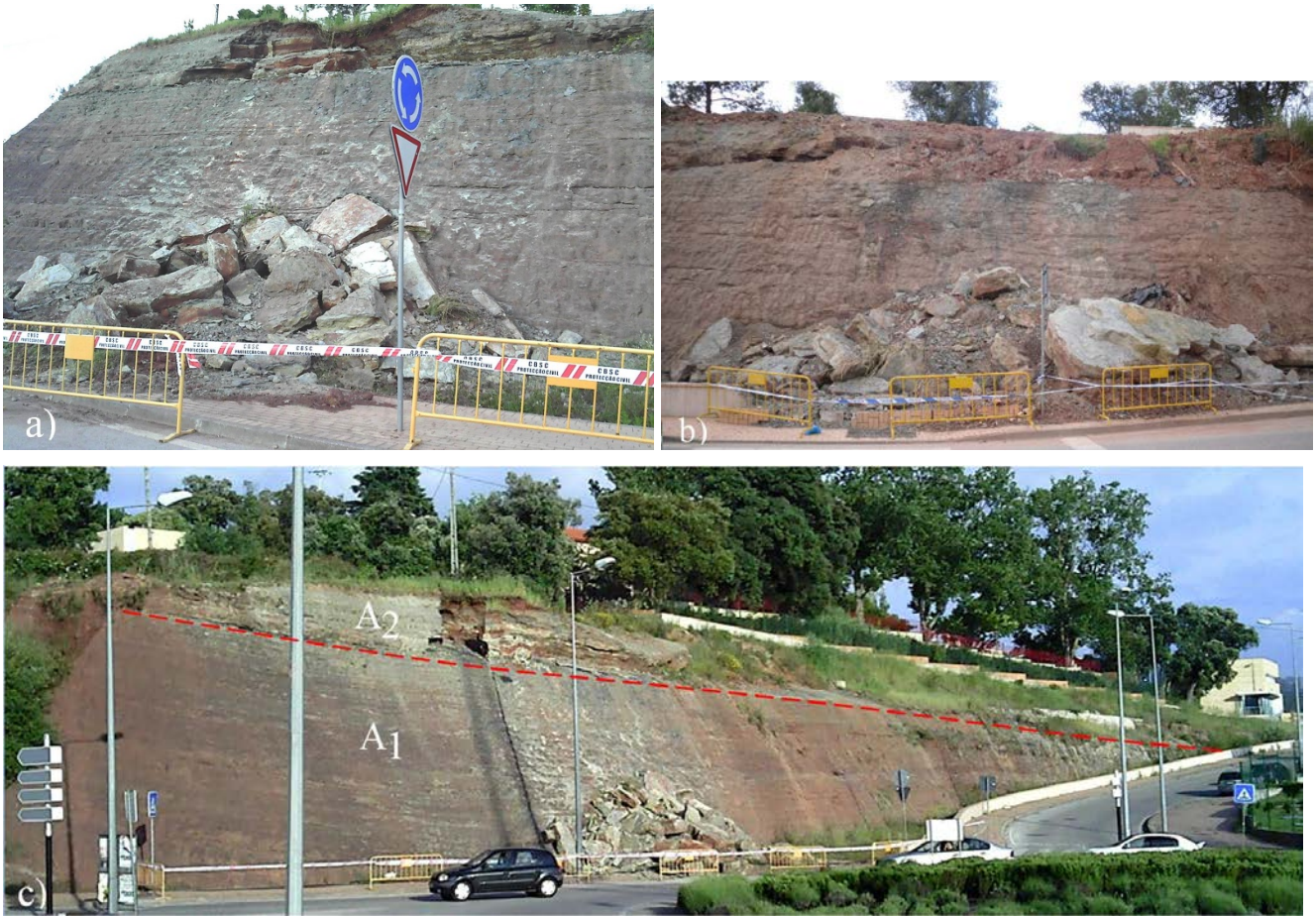
Fig. 7 Areeiro roundabout slope: a May 2011 failure, b April 2010 failure and c global view in May 2011. At left is the Areeiro roundabout slope with accumulation of fallen blocks of the 2011 slide. At centre top, it is visible the scar of the slide surface of 2010. At far right it is visible the Areeiro School slope. The grey mudstone layer responsible for the slides is highlighted by the dashed line. A 1 and A 2 – terms of the “Grés de Silves”
