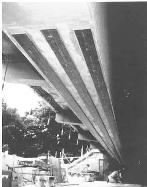
Figure 3.5: Overall view of a concrete beam FRP strengthened on a bridge at Dresden, Germany (Handbook-MIL 17, 2002).
