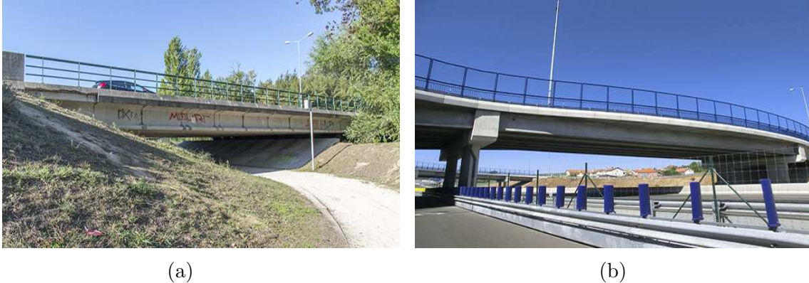
Figure 1.1: PC girders in Leiria over: (a) the pedestrian circuit in the city centre; and (b) highway A19.
