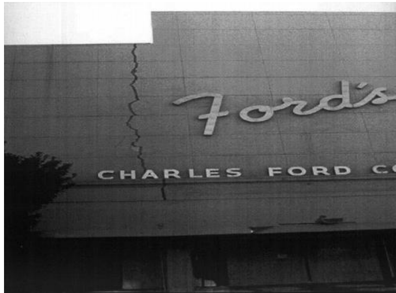
Figure 2.23 – Department Store Façade during Loma Pietra earthquake (EERC)
