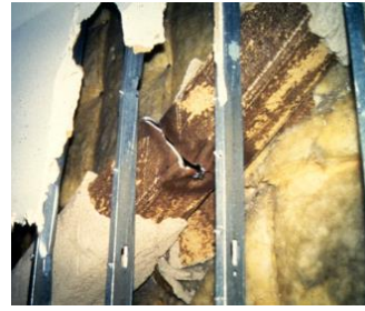
b) HSS brace fracture at mid-length
