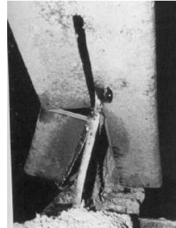
d) HSS brace fracture at net section
