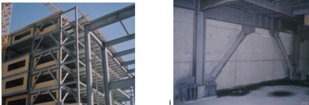
Figure 2.10 – A example of the use of EBF in Istanbul Bilgi University (Turkey) (D'Aniello, 2007)
