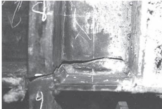
Figure 2.2 – Fracture at the welded beam-to-column connection (Adan and Hamburger, 2010)
