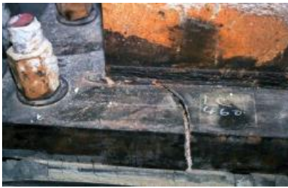
c) Base plate fracture
