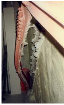
a) Buckled brace
