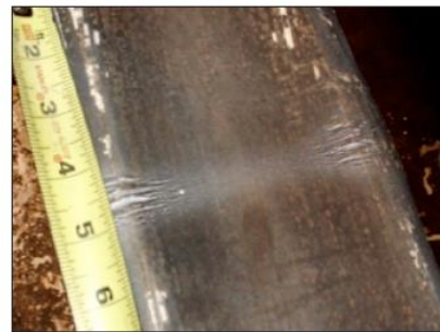
b) Initiation of tearing
