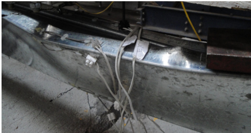
Figure B.32 – Detail view of the failure mode of specimen B-2R_2
