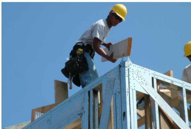
Figure 1.6 – A view of the amount of screws used in connections of CFS structures (Steel Framing Alliance@, 2009)
