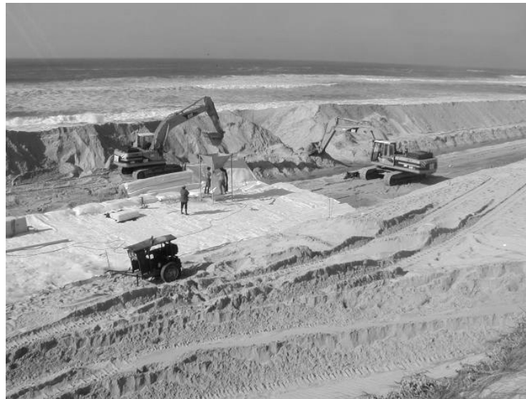
Figure 1.4 – Installation of the sand containers and first layers of geotextiles in the Leirosa sand dune system (Antunes do Carmo, January 2006).
