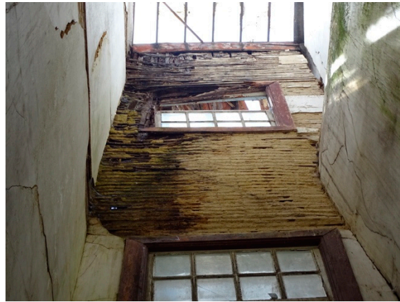
Figure 7. Severely decayed structural elements.
