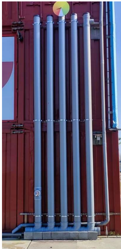
Figure 3.3 - The water wall system in Zernike Campus in Groningen
