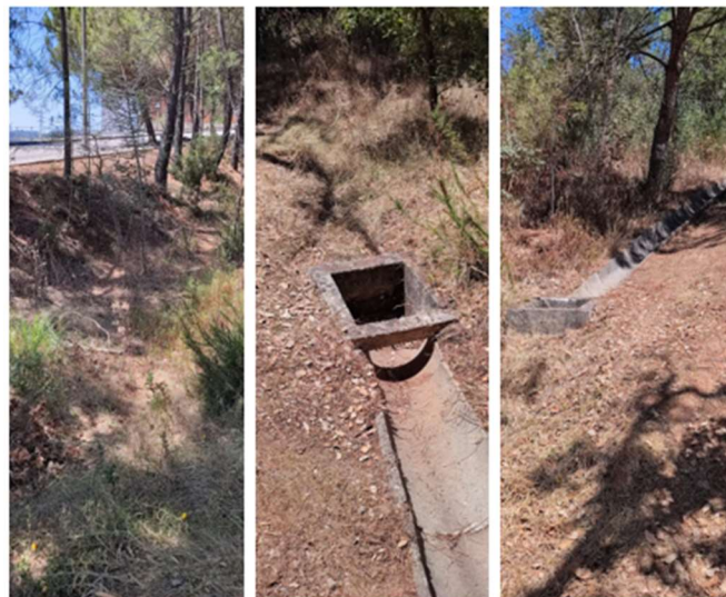
Figure 5.7 - Place of the swale and drainage ditches at FCTUC
