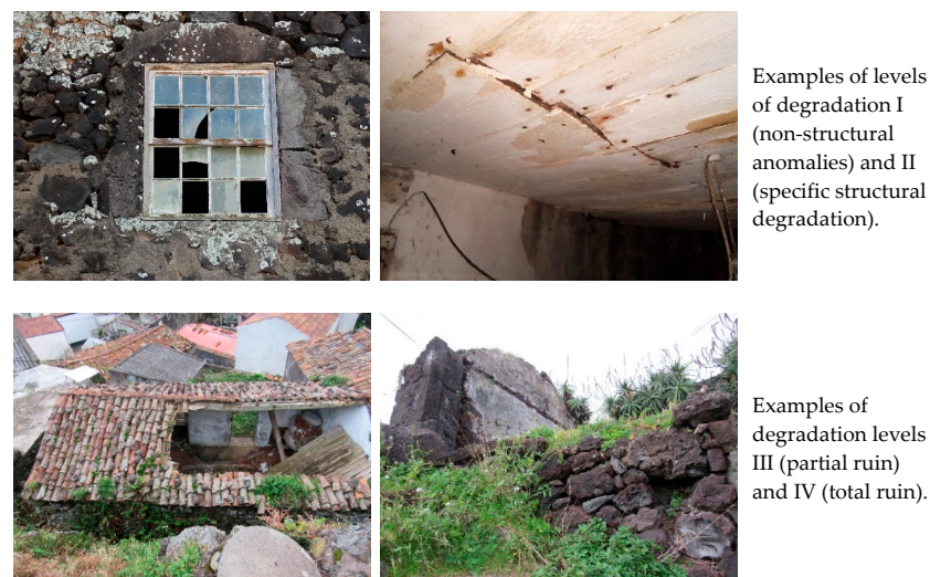
Figure 12. Examples of building degradation situations.
