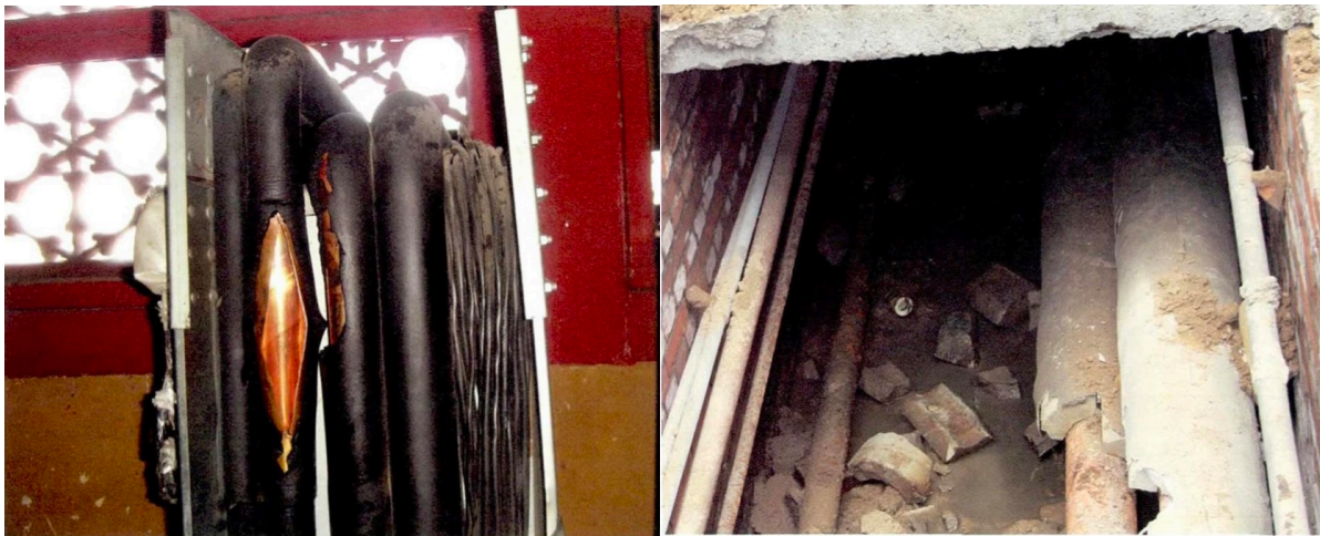
Figure 20 – The Palace Museum's aging infrastructure
