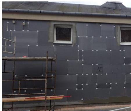
Figure A.4: Real façade using VIP products, applied according to a similar layout pattern planning – Warsaw Zoo.
