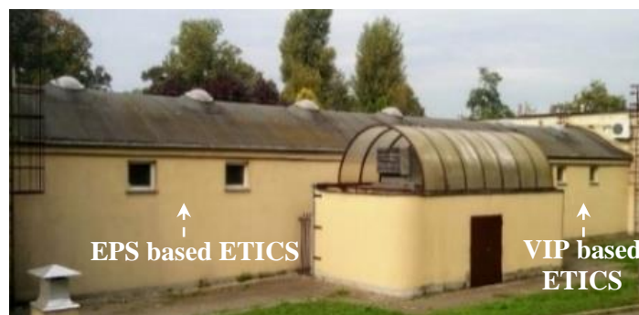
Figure 4.2: Photograph after renovation of the case study façades, including EPS and VIP based ETICS.
