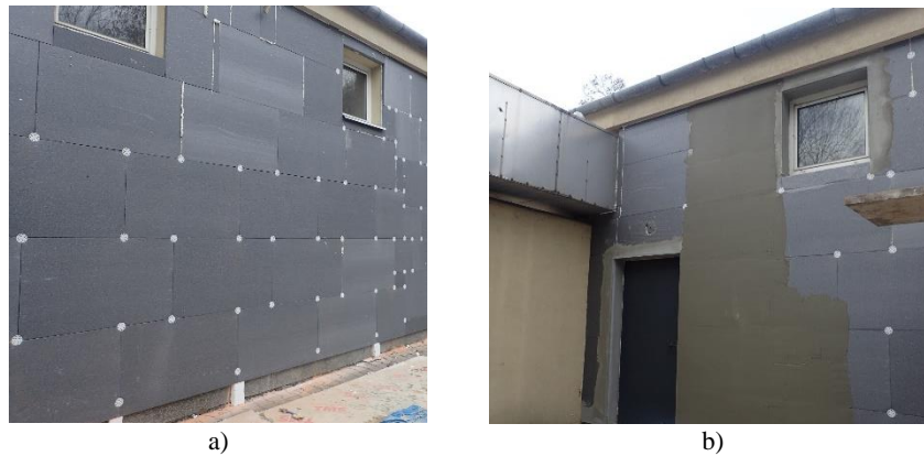
Figure 4.5: Installation of VIP based ETICS: a) encapsulated panels with mechanical fixings at the corners; b) reinforced base coat mortar application.
